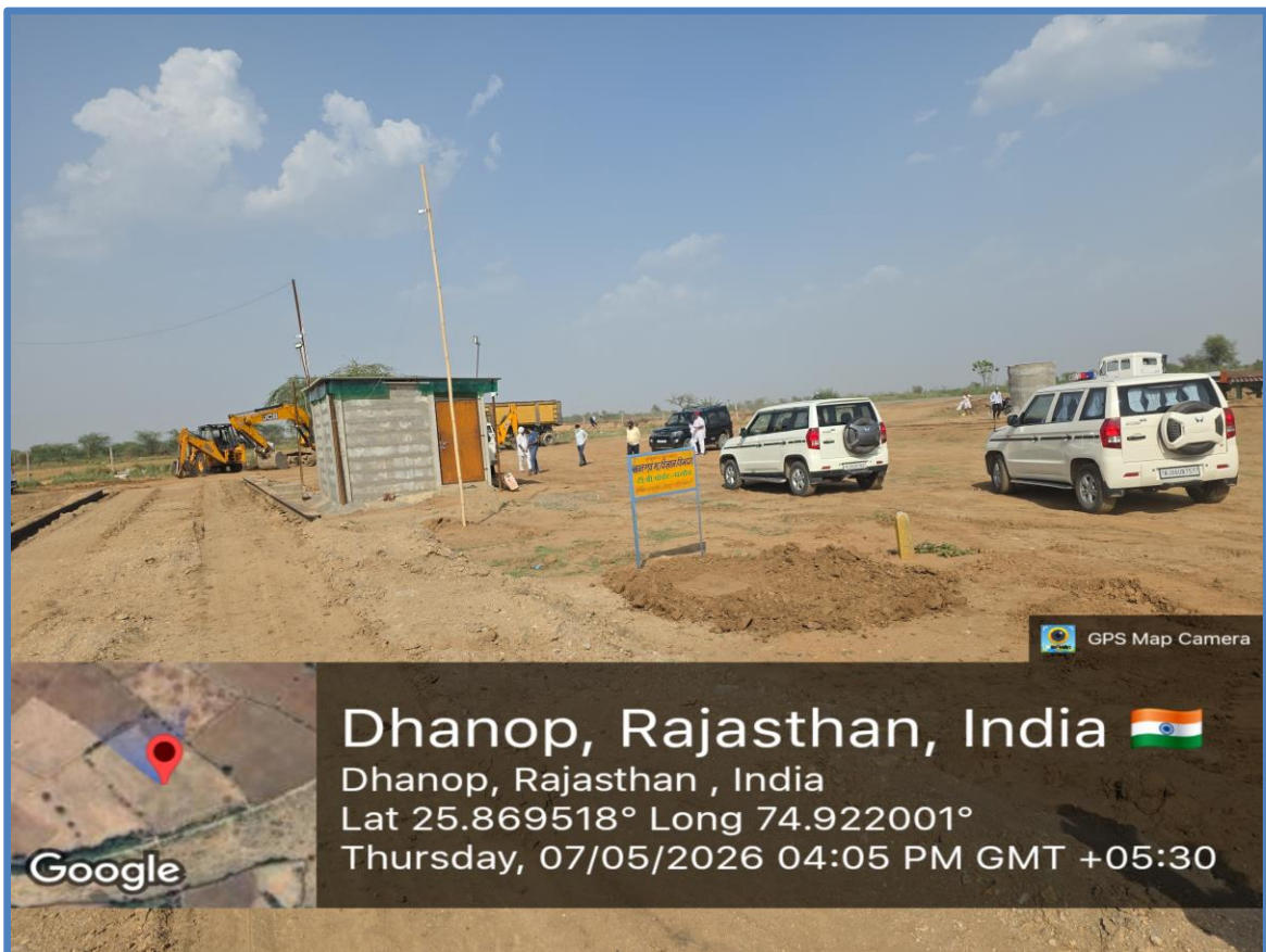
Figure 20: Weighbridge and CCTV installed at Transit Point 02, Dhanop
