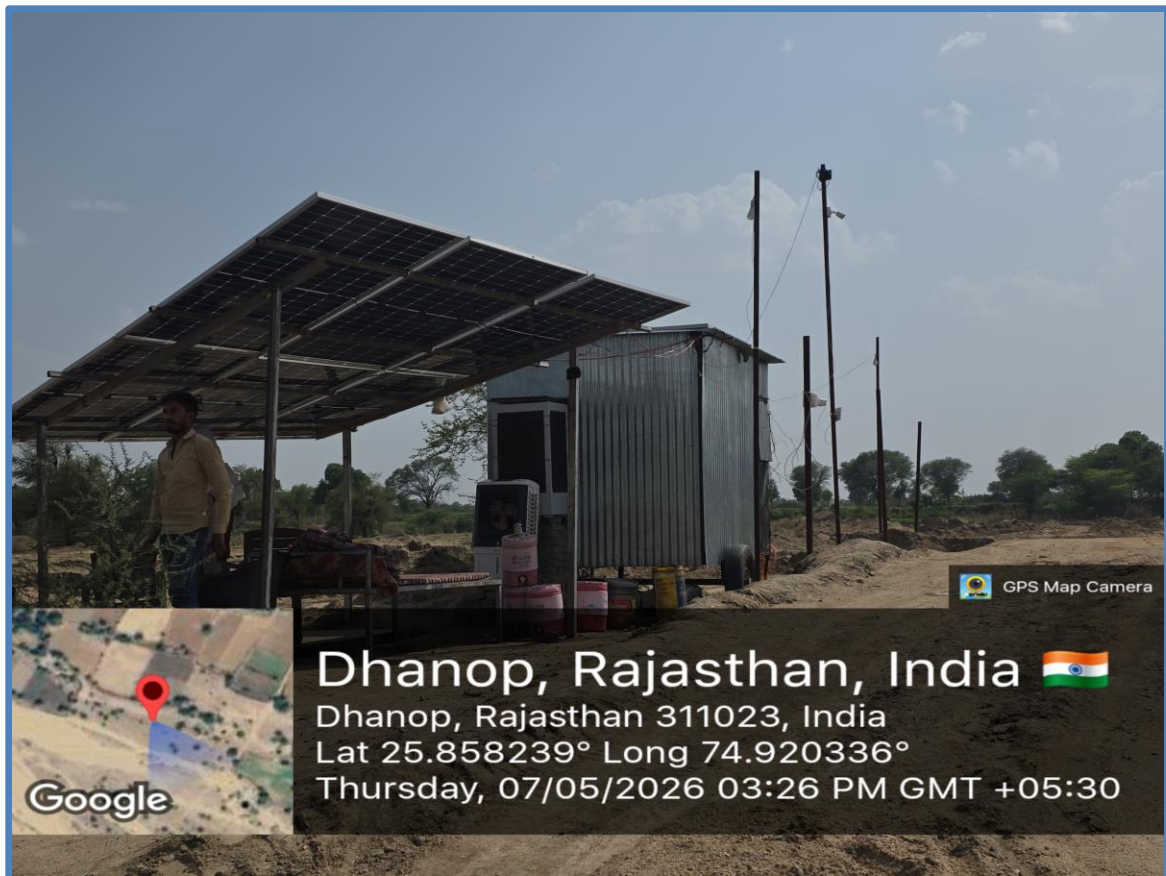
Figure 17: Weighbridge & CCTV Camera Surveillance & Solar plate structure at Khari Riverbed Mining area, Dhanop Mining Point 1
