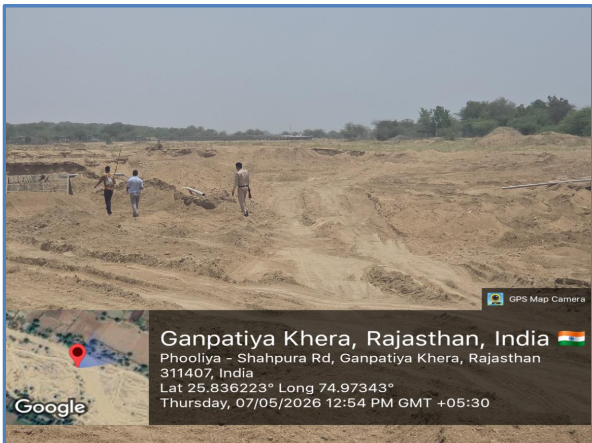
Figure 6: River sand mining sign at Khari Riverbed
