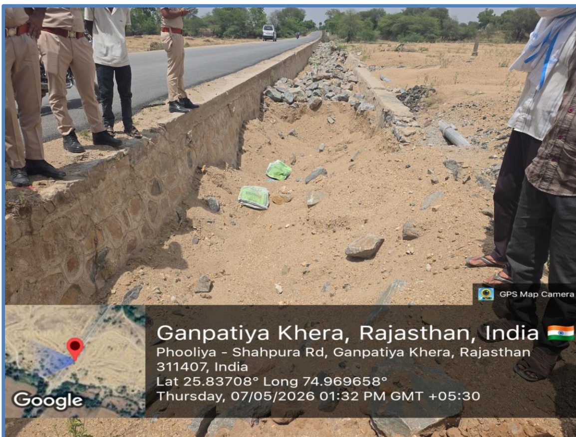
Figure 11 : Shallow mined section(minor excavation) along the Raod passing through Riverbed at. The Joint Committee immediately directed the lessee to backfill the area to restore its integrity at Phooliya Kalan Riverbed section (Towards Singari)
