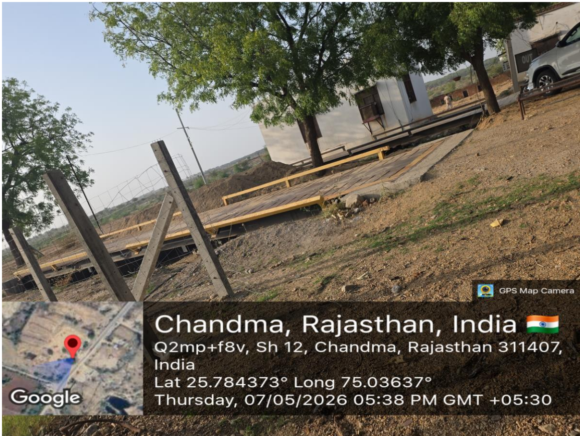
Figure 25: Weighbridge & CCTV Camera Surveillance at Khari Riverbed area, Badla Transit Point 03
